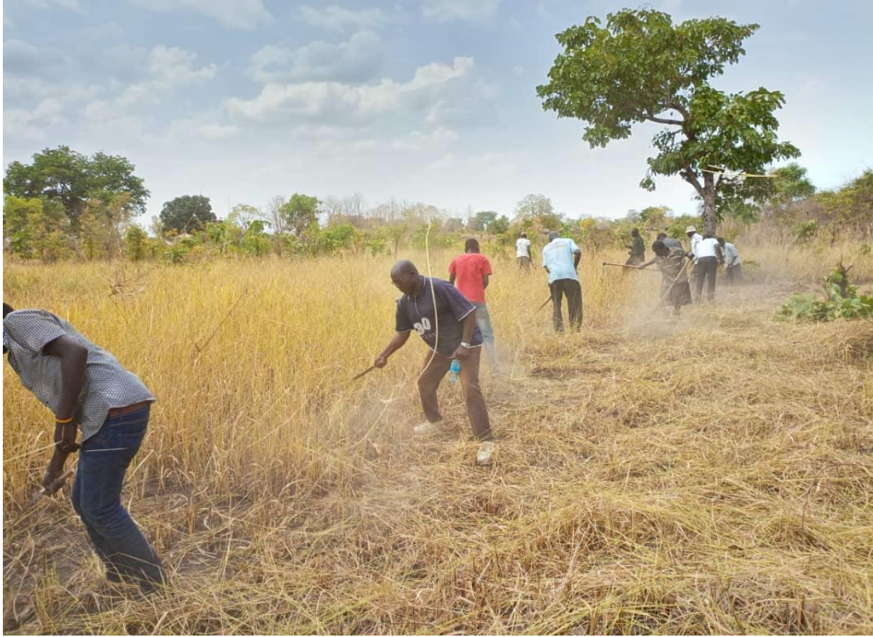
'Buagyi Community at work preparing the construction site for the 'Buagyi Maternity Center. This is a community self-help initiative.
